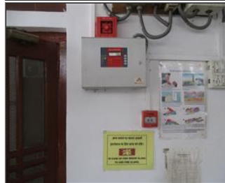
Photo of fire safety equipment Centralised Fire Alarm Panel.JPG
