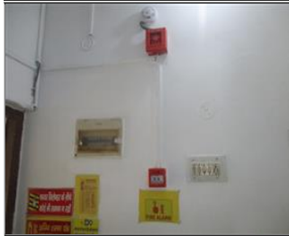
Photo of fire safety equipment Fire Alarm Call Point Hooter and Smoke Detector.JPG
