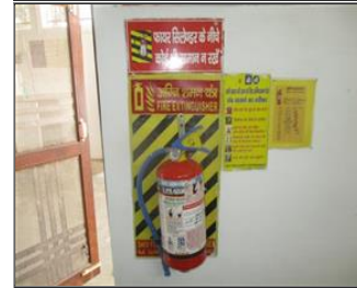
Photo of fire safety equipment Fire Extinguisher.JPG
