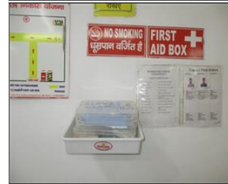
Photo first aid facilities First Aid Box.JPG
