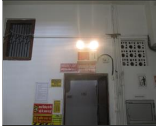
Photo of fire safety equipment Emergency Light Tested.JPG
