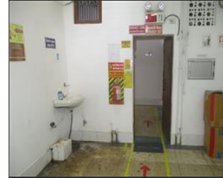
Photo of fire safety equipment Exit with Emergency Light.JPG
