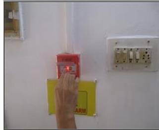
Photo of fire safety equipment Fire Alarm Call Point Tested.JPG
